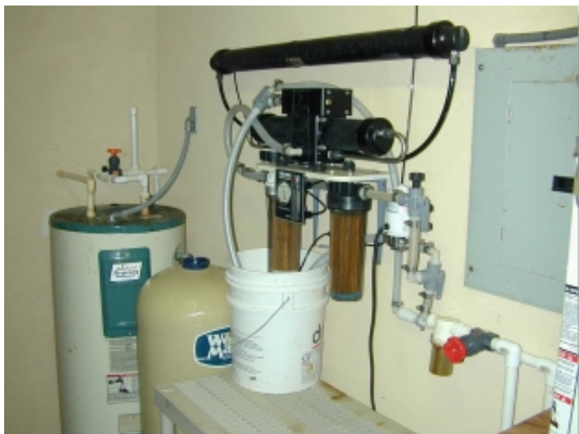
Land Based Installation
